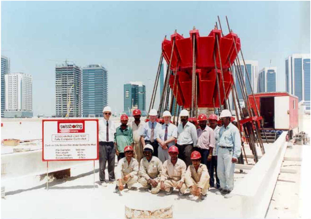
Site of large-capacity pile load test for the Emirates Towers in Dubai in 1997. Poulos is fourth from left in back row. (Photo by H. Poulos.)
