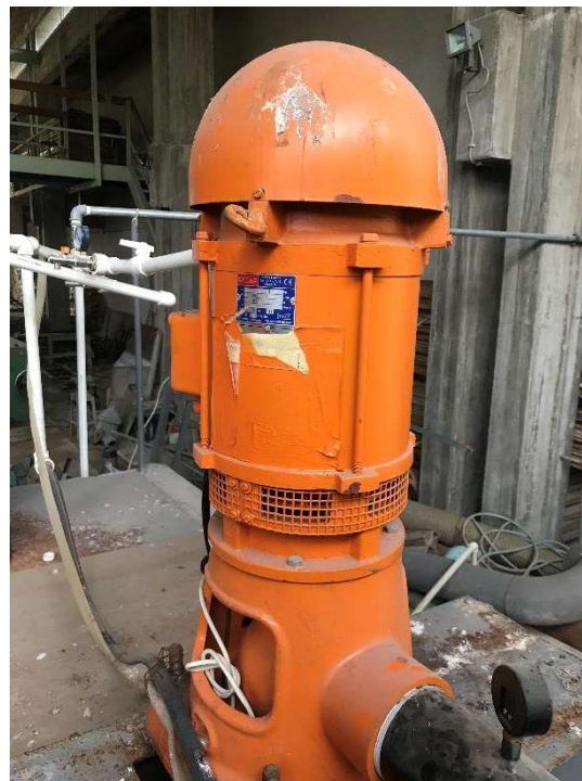
Pump (50 lt/sec) One of the pumps supplying water for the Hydraulic Laboratory
