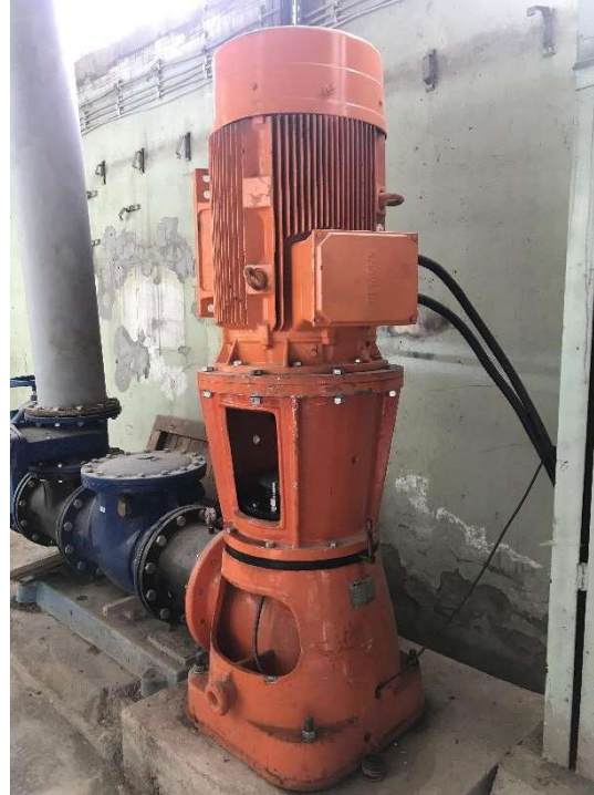
Pump (250 lt/sec) One of the pumps supplying water for the Hydraulic Laboratory
