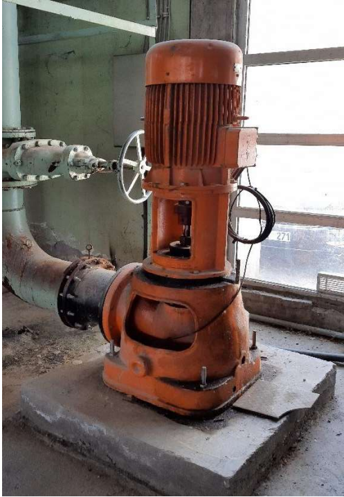
Pump (125 lt/sec) One of the pumps supplying water for the Hydraulic Laboratory
